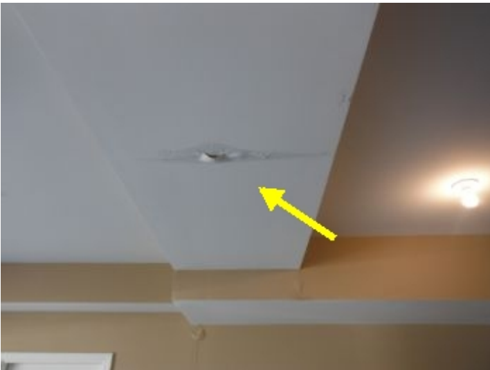
water leak for jetted tub
