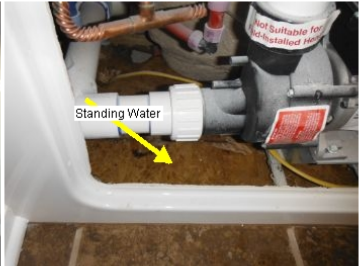
Water leaking under jetted tub, Standing water Was Under tub
