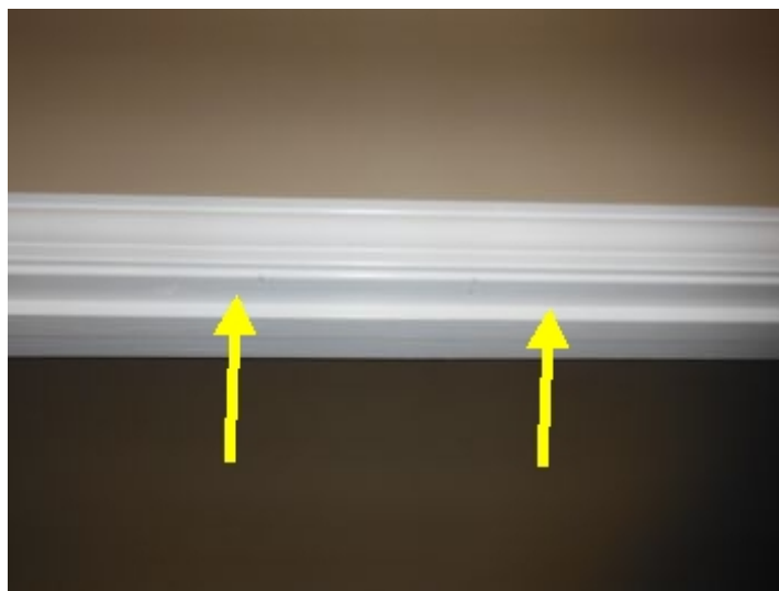
Latch Plates not installed on Closet door(s),
