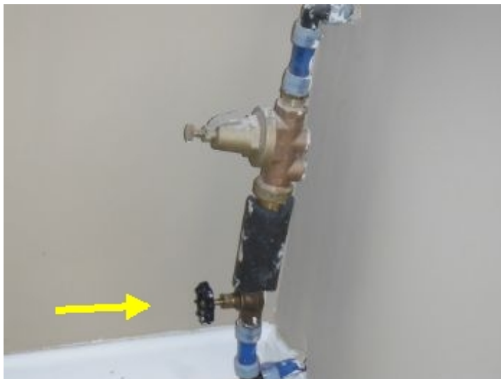
water shut off valve
