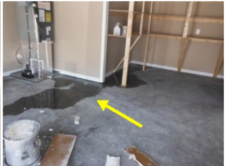
water leak from jetted tub
