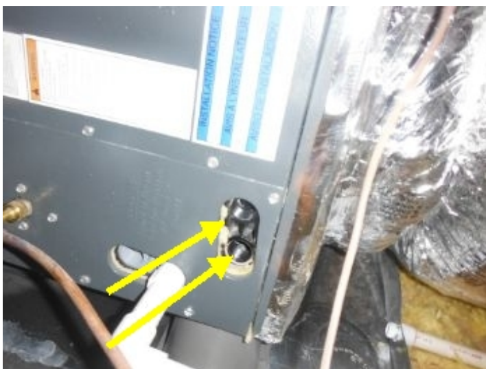
Missing drain plugs on the attic a/c unit
